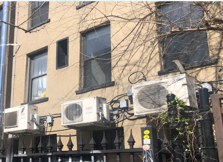
Outdoor Heat Pumps
