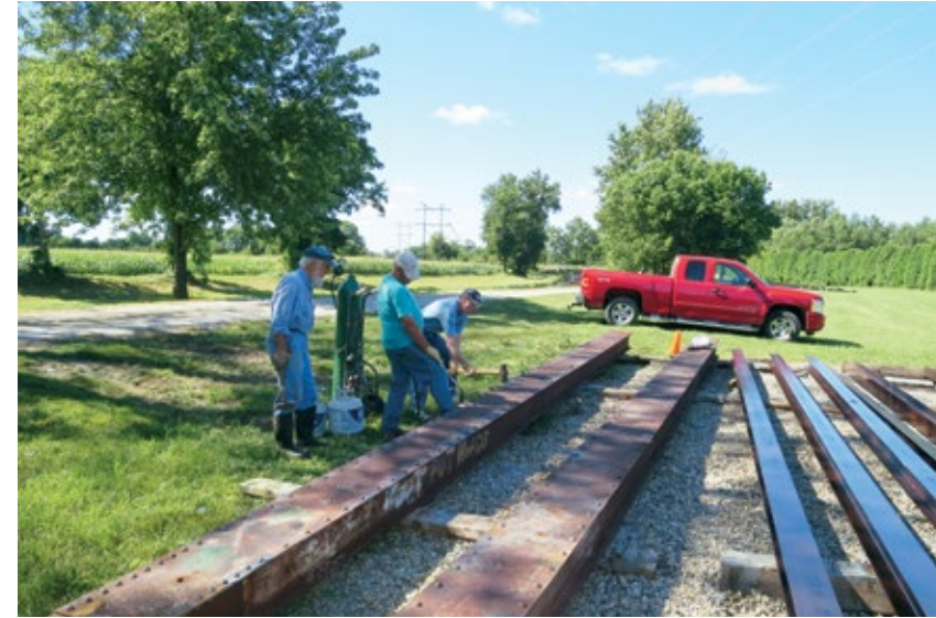
The Monday-Wednesday-Friday Crew hammers down rivets on iron girders, pieces of the Gray Bridge, which was disassembled, reworked, and which is now being reconstructed in the city of Delphi.
